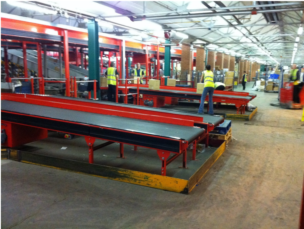
Heavy duty Belt Conveyor (Belt on Deck) being loaded cases of wine (see above photo) and general parcels (see photo below),in service since 2010 7 days a week.
